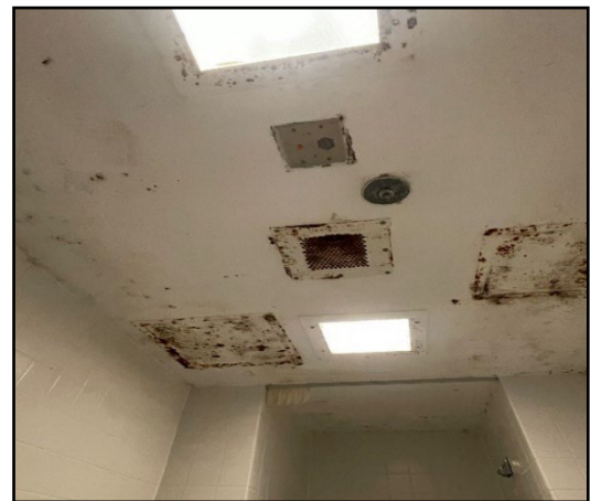
Figure 8. Mold on shower ceiling, March 2025.
